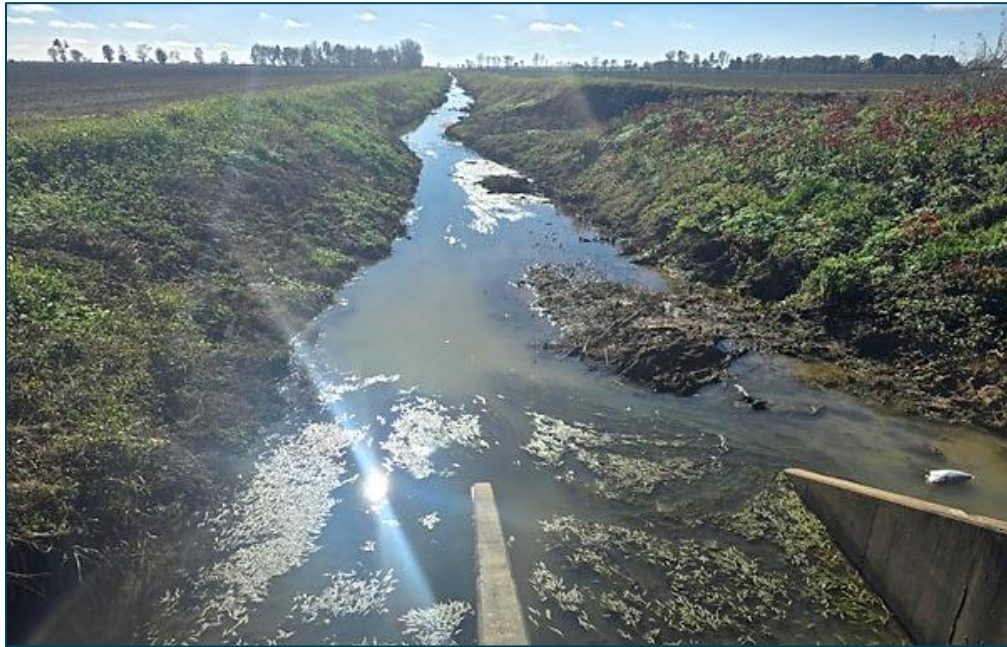
Photo: Erosion on Main Ditch, Conservation Works Joint Venture Partner 11/20/2024
