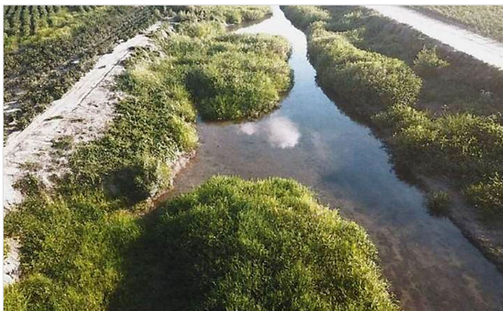
Photo: Erosion on West Ditch – Main Ditch, Conservation Works Joint Venture Partner November 2024
