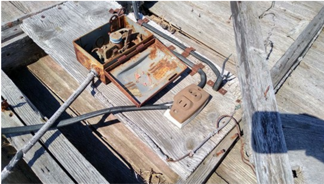
Figure 26. Destroyed Pumphouse Electrical Installation
