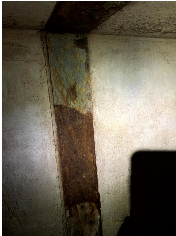
Photo 45: Steel plate corrosion, Joint #18.
