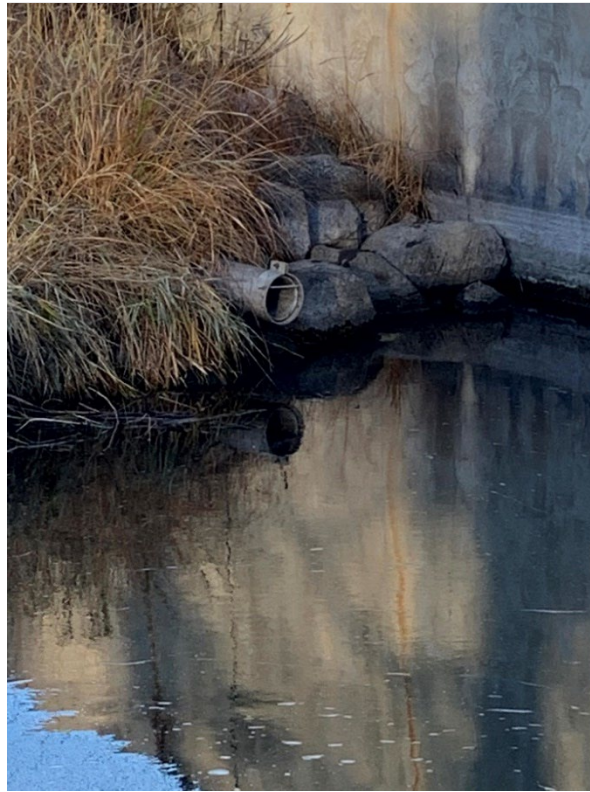
Photo 8: Right foundation drain outlet, missing animal guard.
