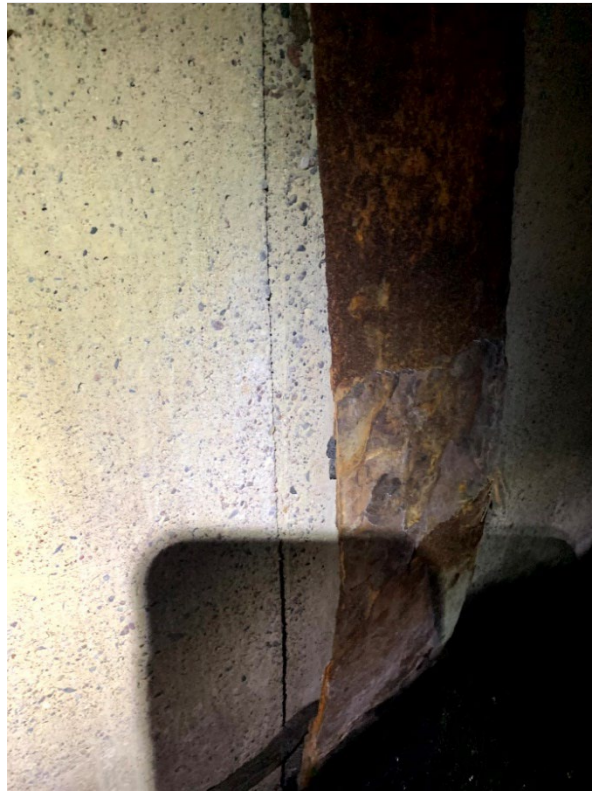
Photo 35: Separated steel plate, Joint #8.
