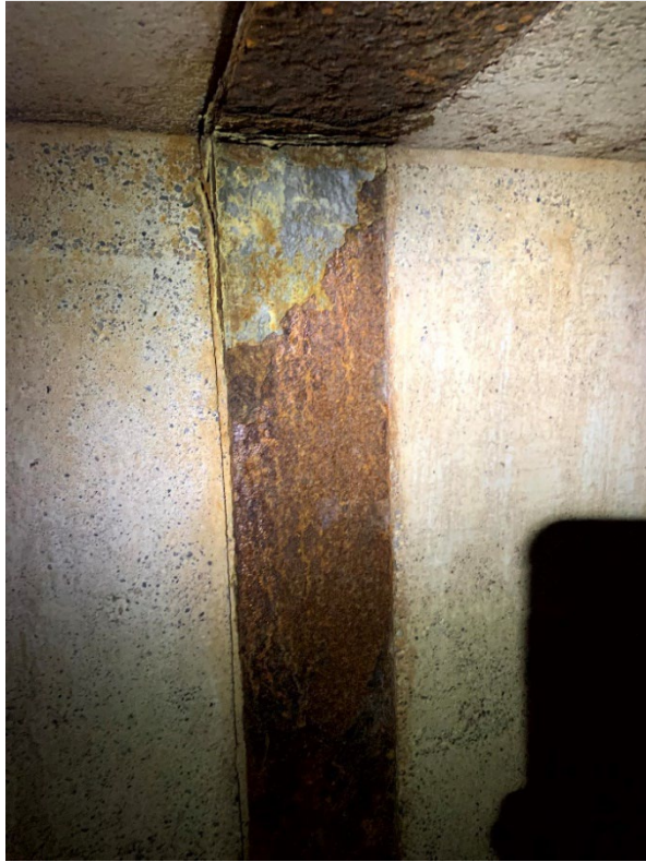
Photo 36: Steel plate corrosion, Joint #9.
