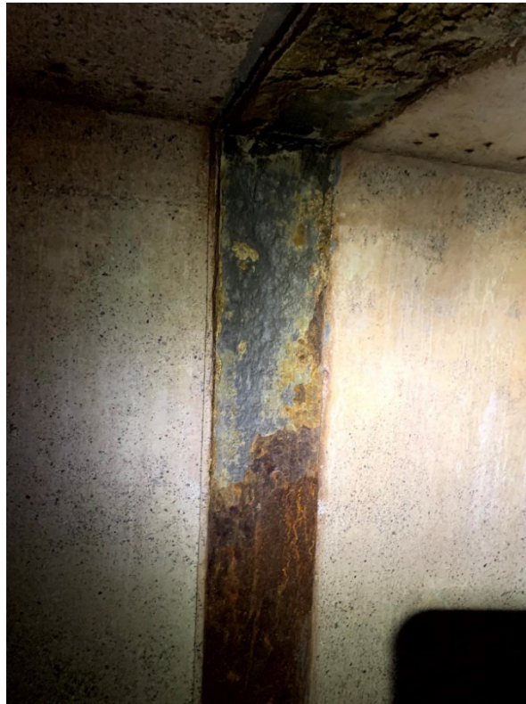
Photo 39: Steel plate corrosion, Joint #12.
