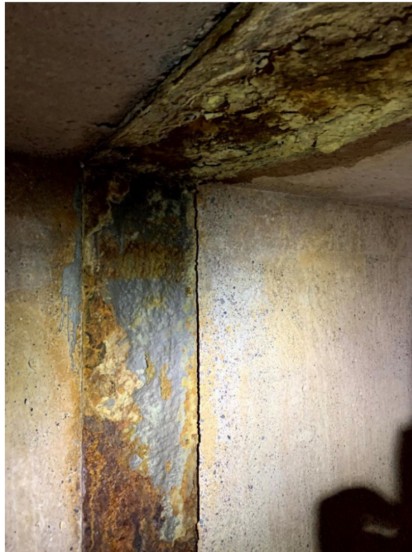
Photo 31: Steel plate corrosion, Joint #4.
