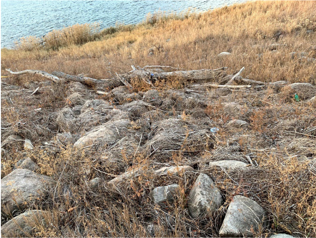
Photo 11: Debris on upstream slope.
