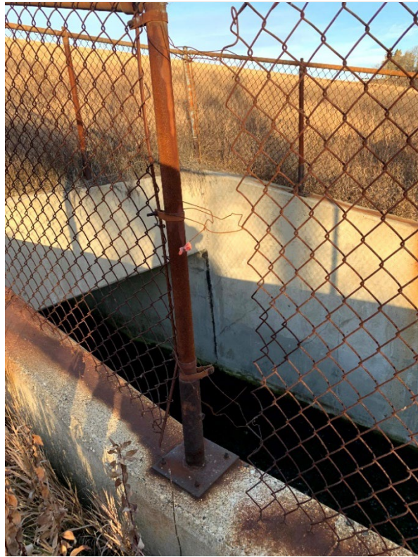
Photo 3: Gap in chain link fence of principal spillway outlet.
