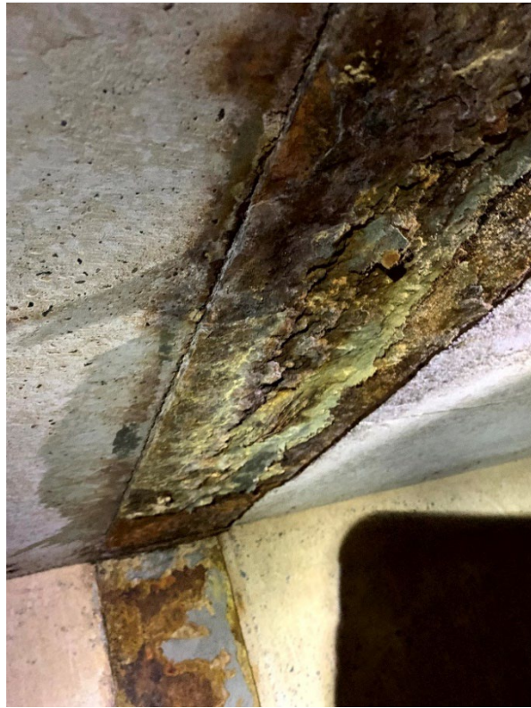
Photo 41: Steel plate corrosion and wet on top, Joint #14.
