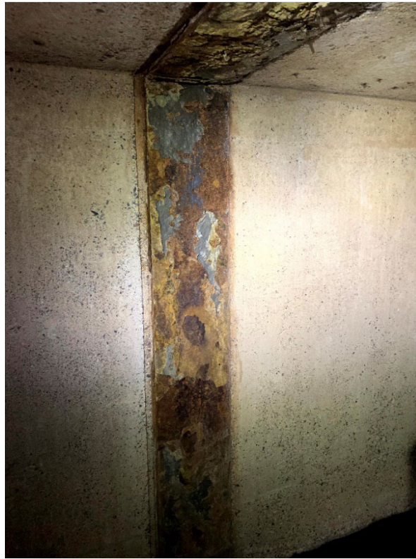
Photo 40: Steel plate corrosion, Joint #13.
