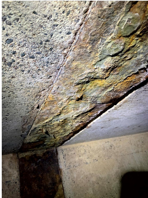
Photo 42: Steel plate corrosion, Joint #15.
