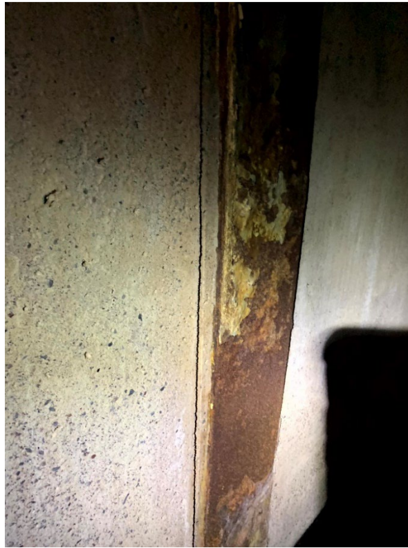
Photo 34: Separated steel plate, Joint #7.
