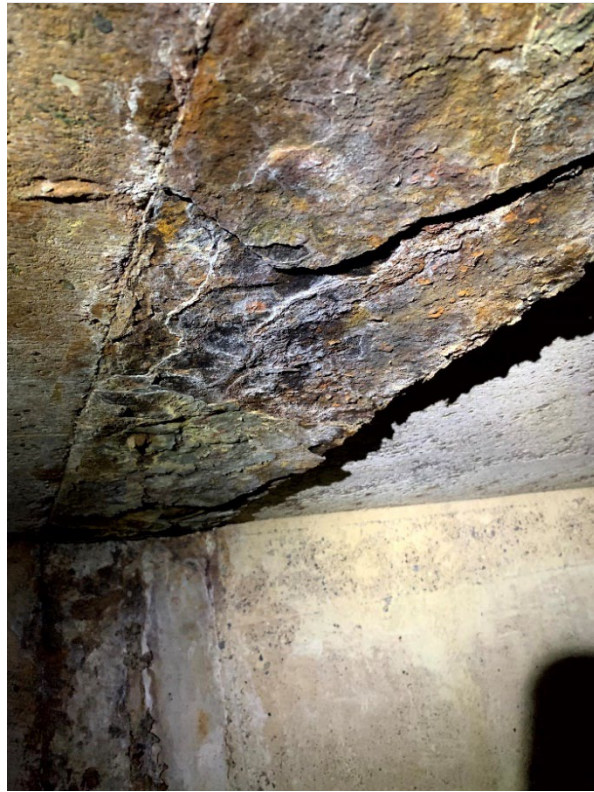
Photo 44: Steel plate corrosion and missing plate, Joint #17.
