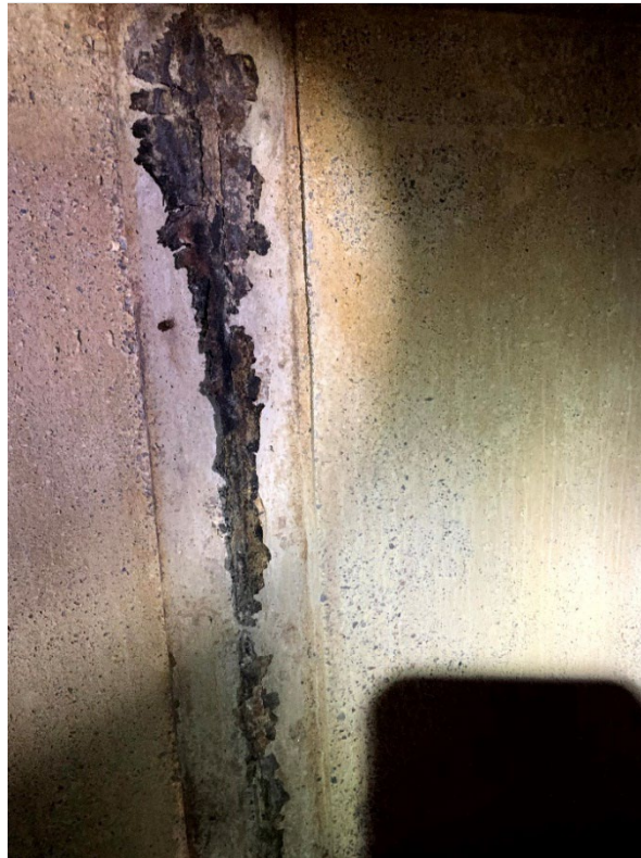
Photo 33: Missing steel plate, Joint #6.
