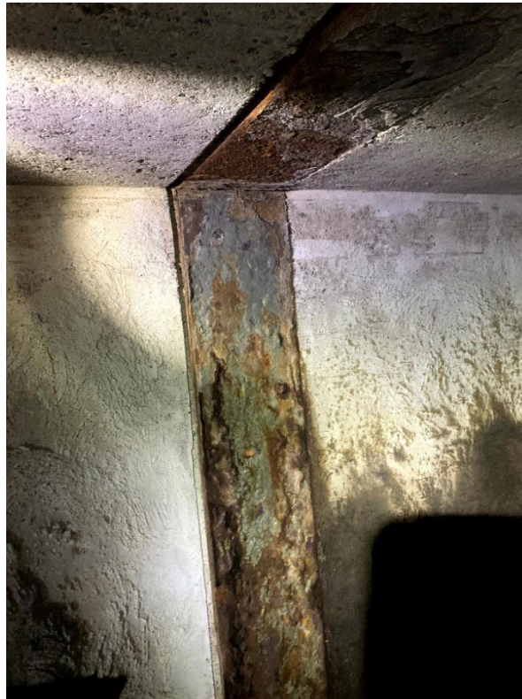
Photo 46: Steel plate corrosion, Joint #19.
