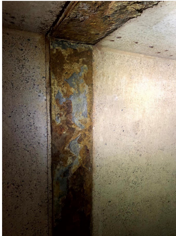
Photo 37: Steel plate corrosion, Joint #10.
