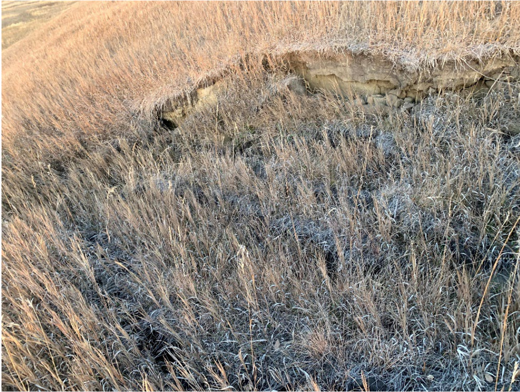
Photo 27: Erosion/slough in left side slope of auxiliary spillway.
