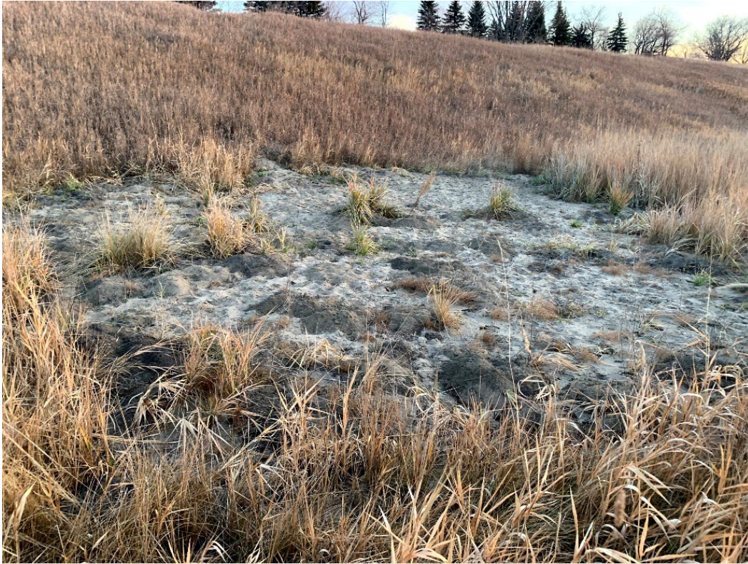
Photo 26: Gopher mounds, auxiliary spillway.
