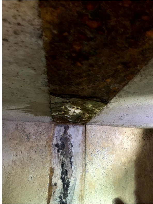
Photo 32: Missing steel plate, Joint #5.
