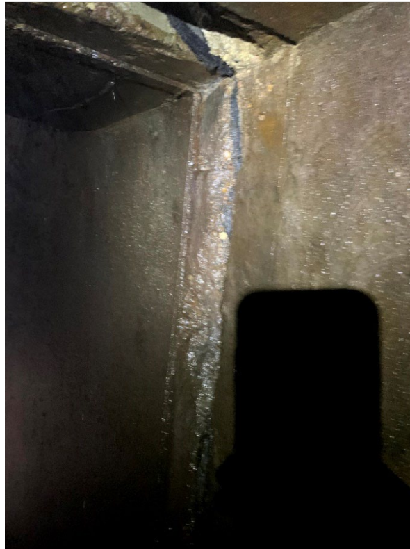
Photo 47: Missing steel plate, Joint #20.
