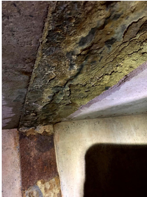
Photo 38: Steel plate corrosion, Joint #11.
