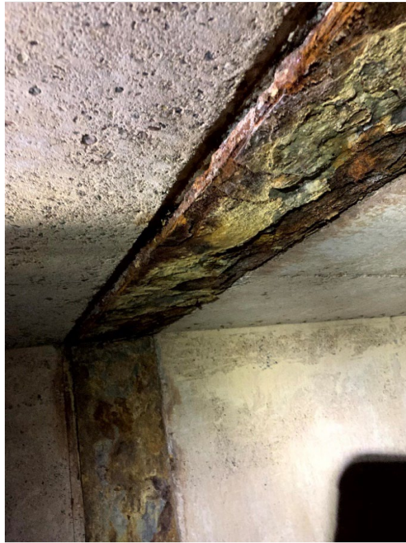
Photo 43: Steel plate corrosion, Joint #16.
