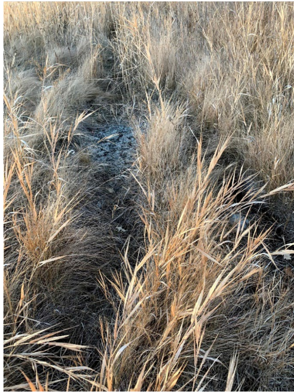
Photo 16: Rutting on downstream berm.
