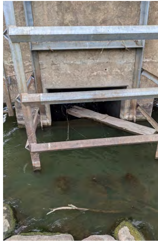
Figure 20 Larimore Dam Primary Inlet with trash
