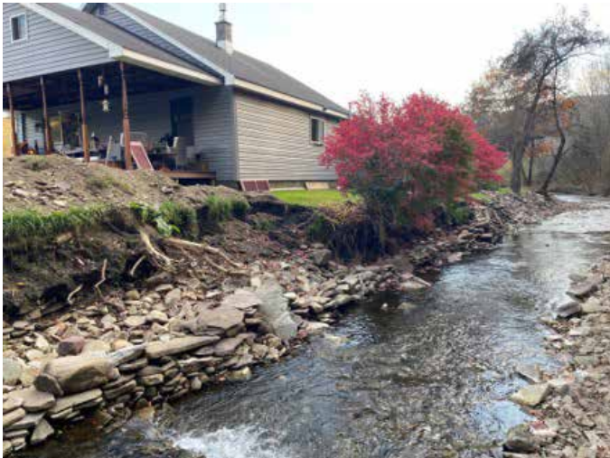
Before: A major storm severely eroded the streambank near this house.
