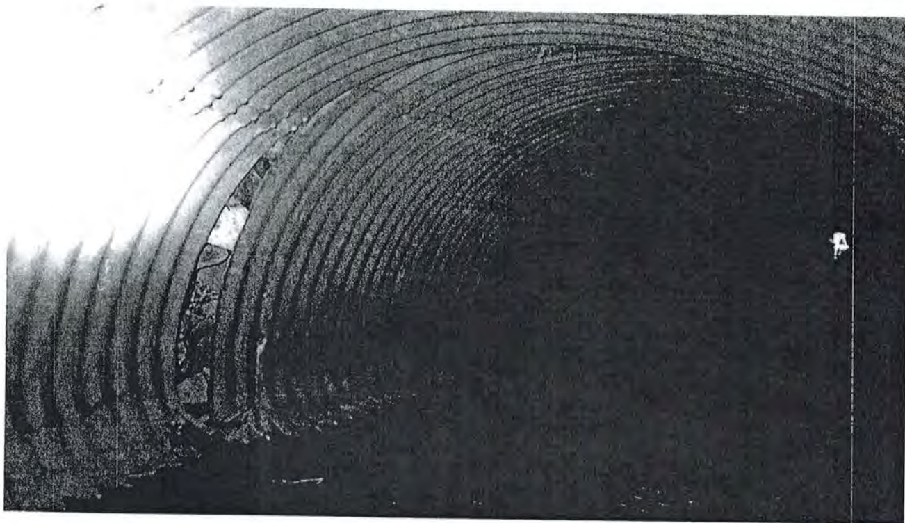
Figure 6: Poor Pipe Splice Transition at 100 feet.
