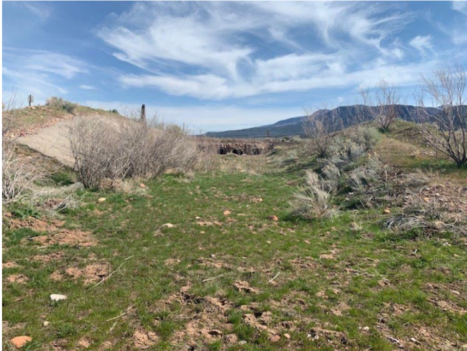
Figure 3-6: Willows Growing in the Emergency Spillway Intake (DWRi 2023b)
