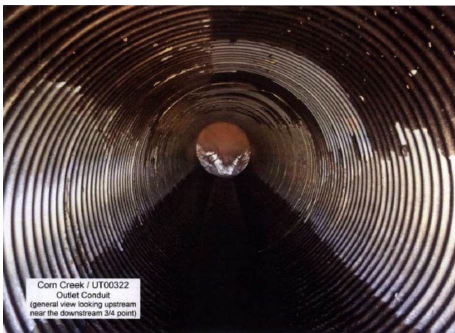
Figure 3-8: 60-inch Conduit (DWRi 2019)
