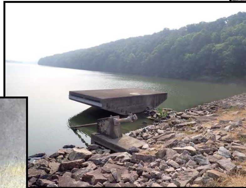
PSW Riser & Pond Drain
