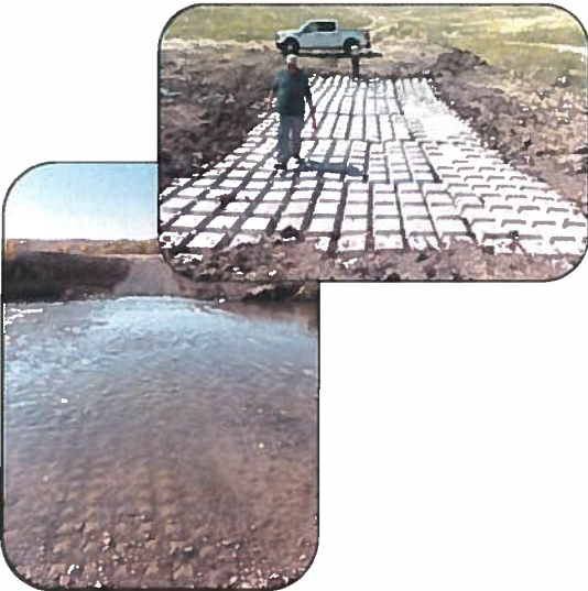
Stream Crossing: Articulated Cable Concrete Blocks and Mats
