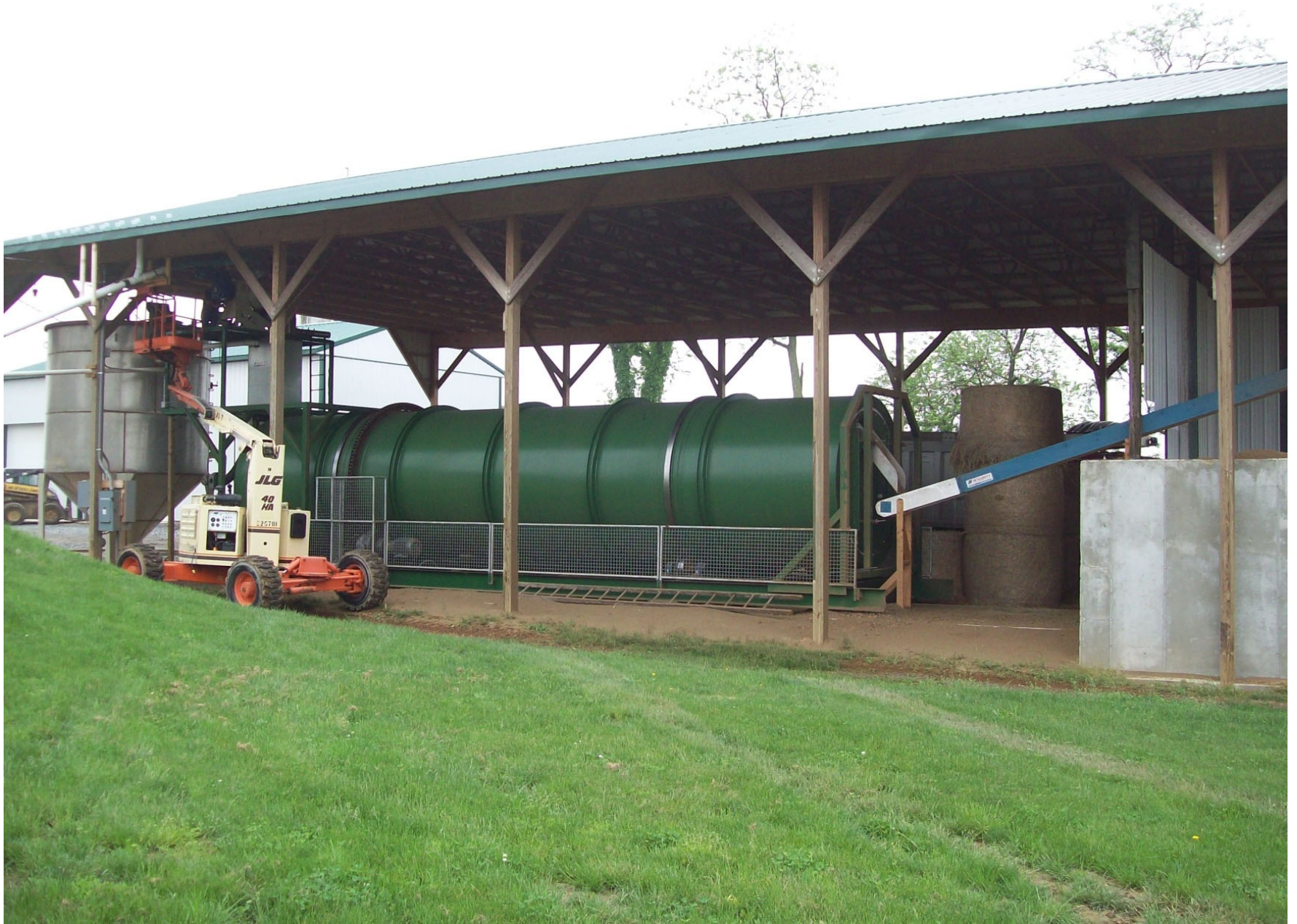
Drum Composter to treat and dry manure solids
