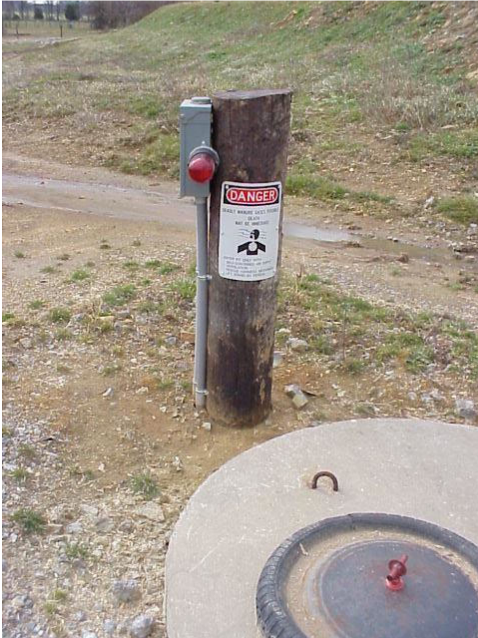
Leachate pump tank with warning light
