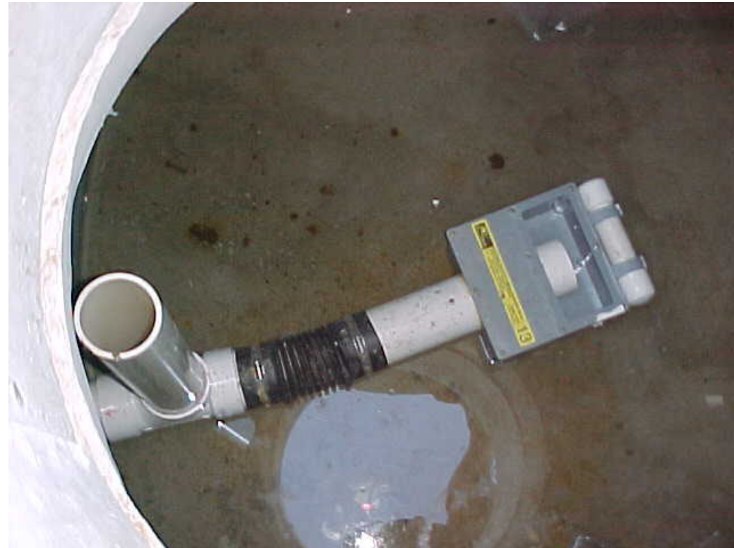
Collection tank with Flout to control discharge
