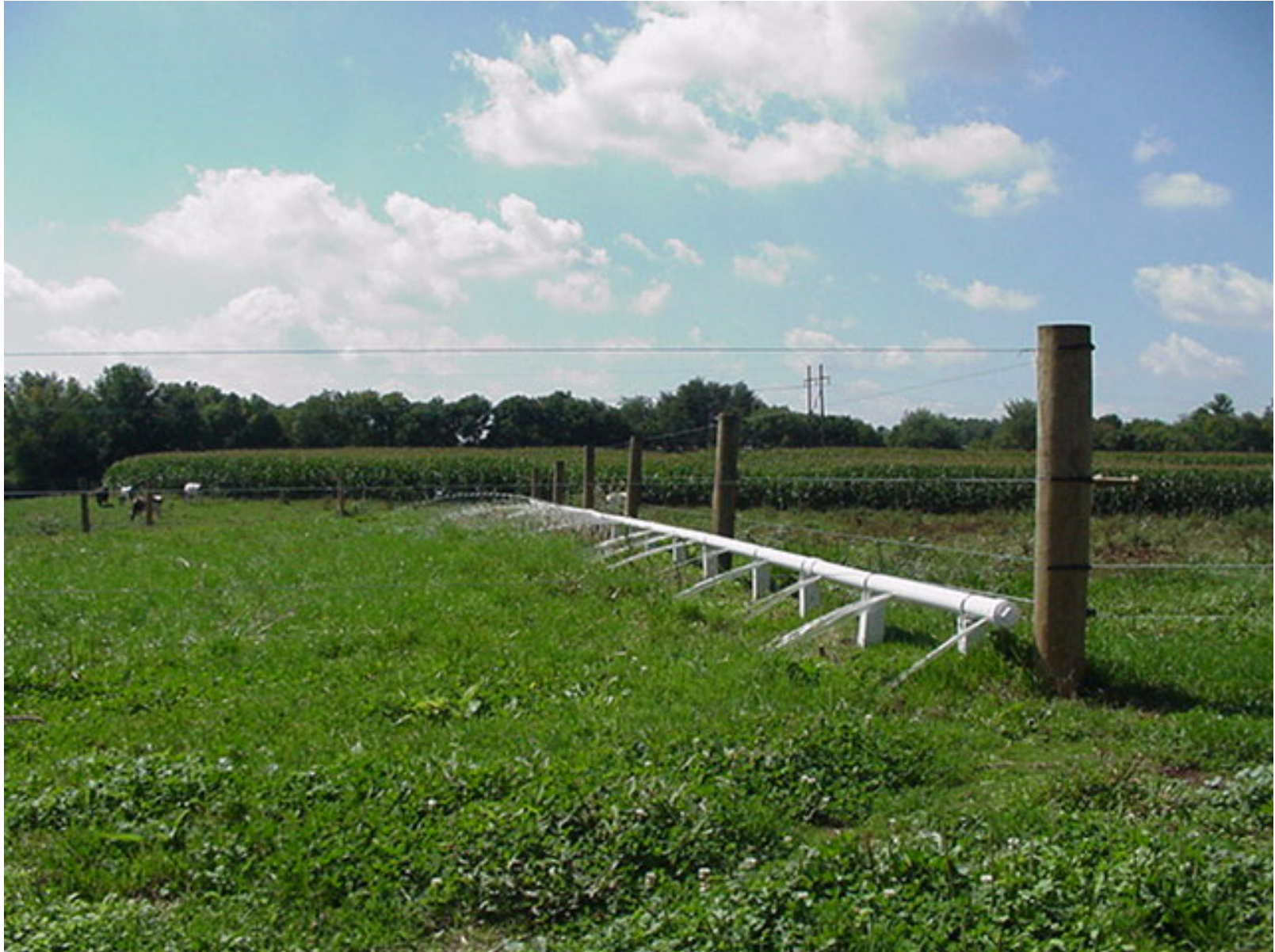
Spreader pipe distribution system above waste treatment strip
