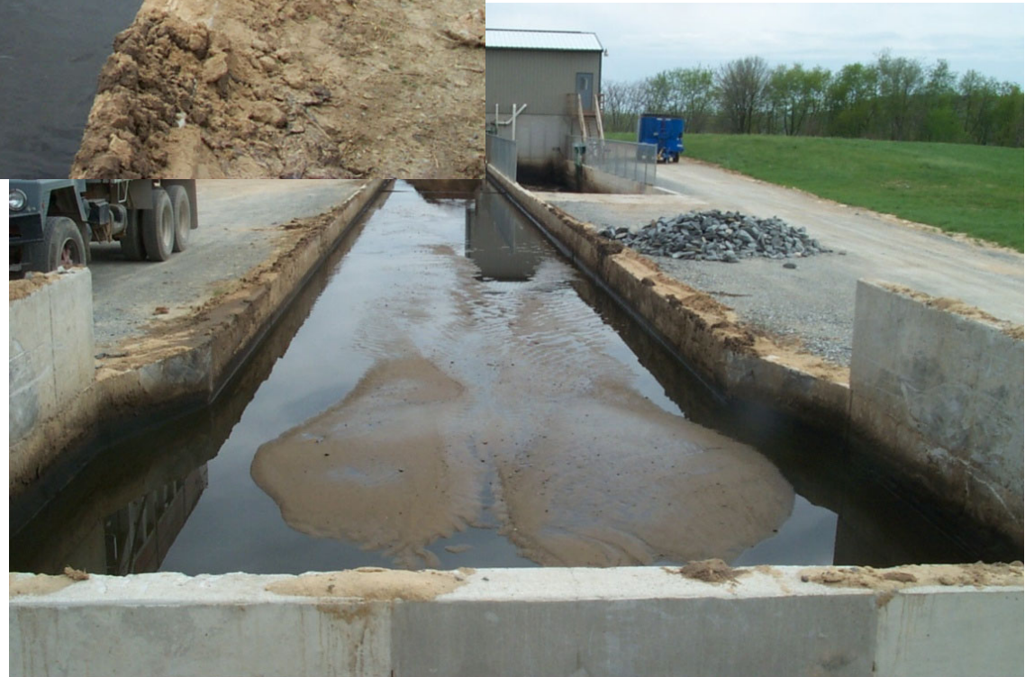
Sand settling lane looking downstream at end of flush
