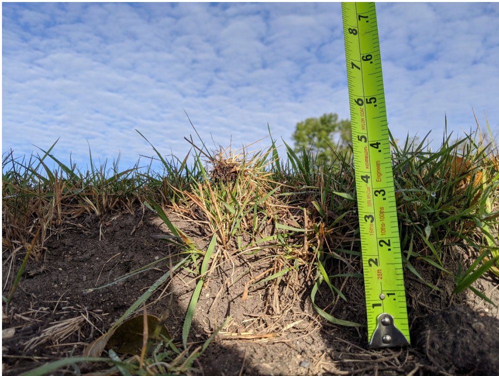
Photo 8 – rutting depth on crest
