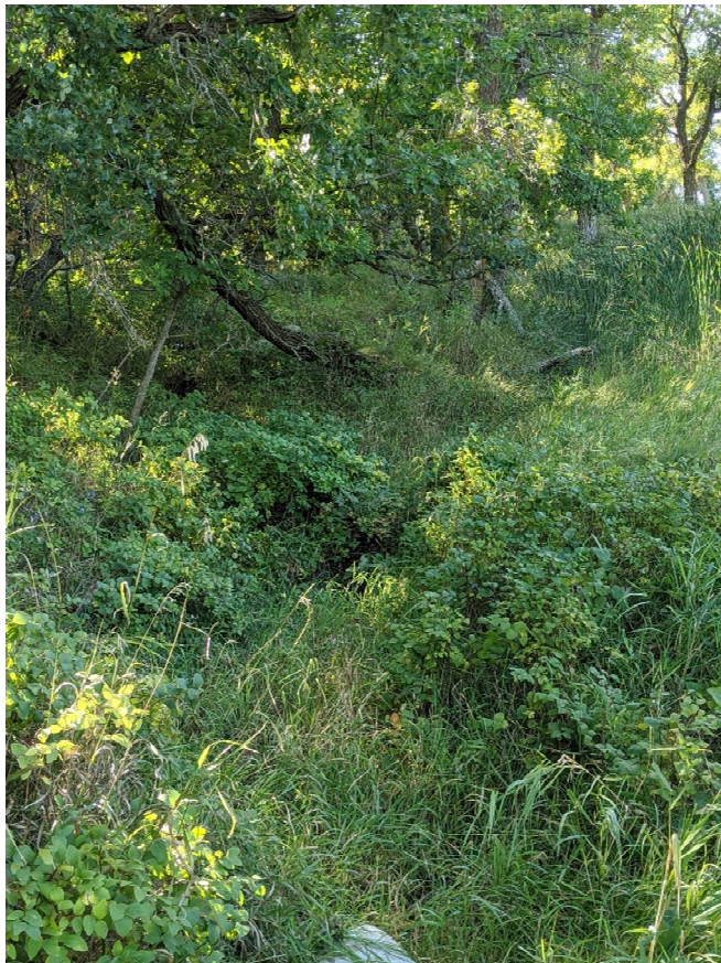
Photo14 – active erosion on downstream right groin looking S
