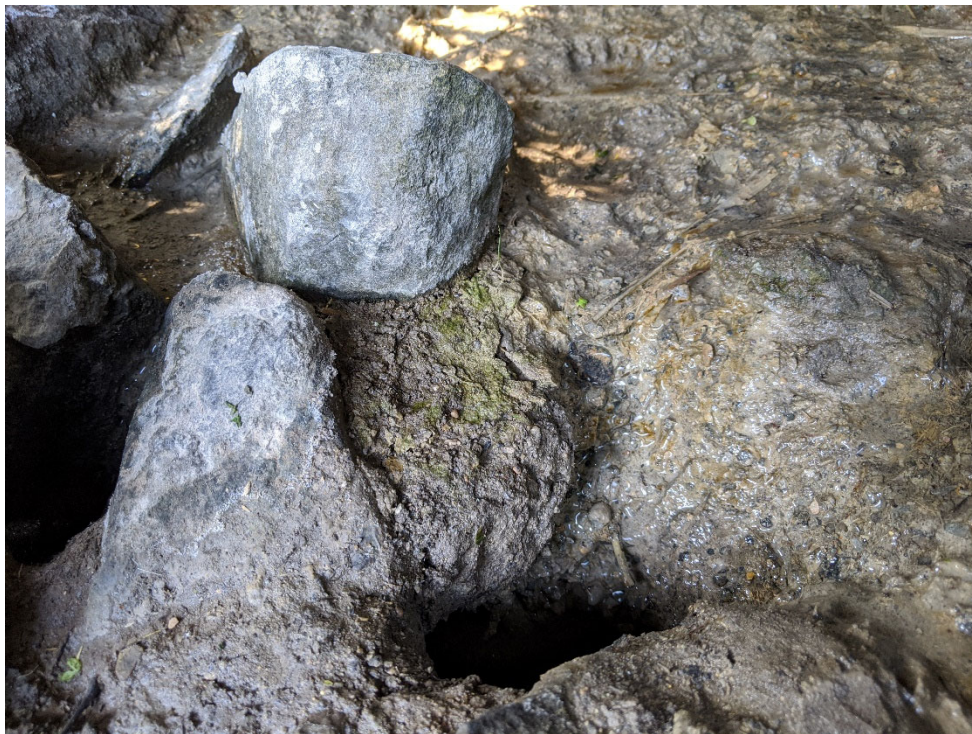
Photo 24 – visible flow directly under principal spillway conduit at outlet
