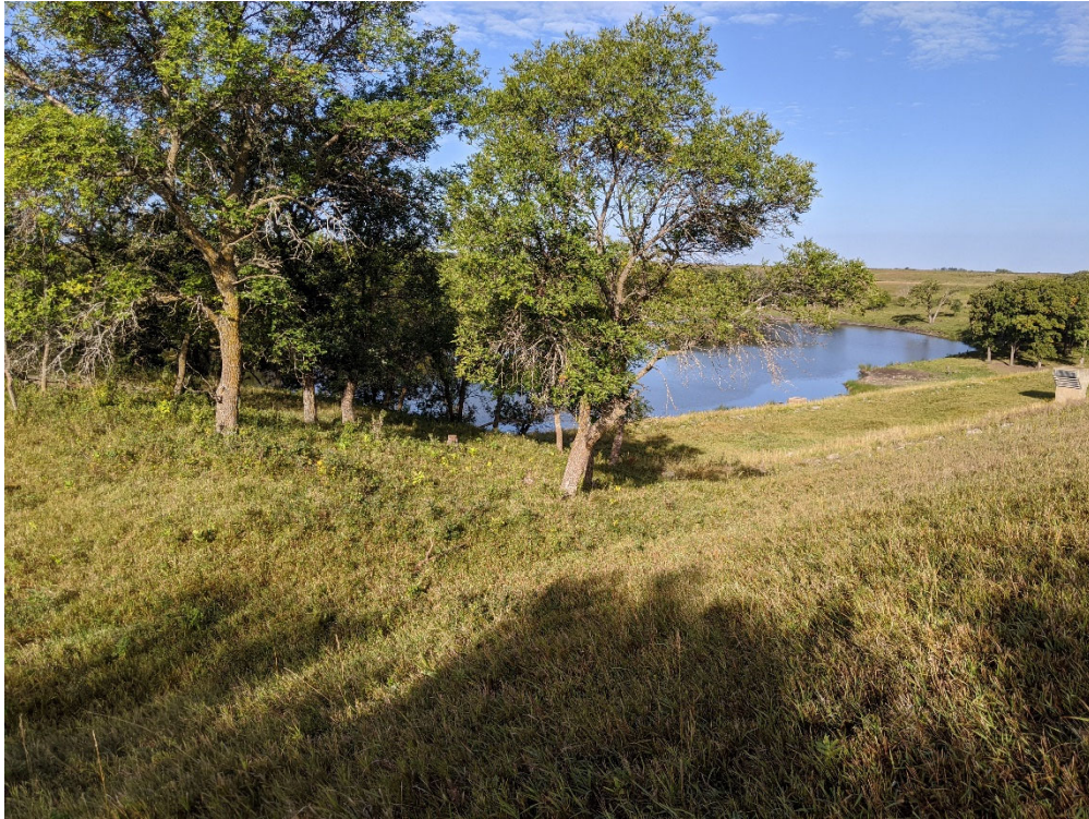
Photo 11 – tree encroachment on right upstream abutment looking W
