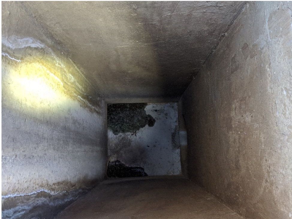
Photo 2- low-stage riser vault
