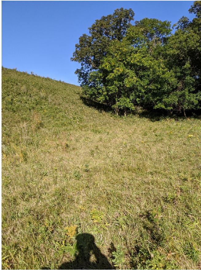
Photo 13 – encroachment on left abutment looking N
