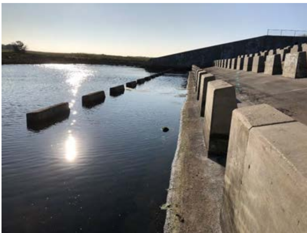
Photo 6 Bottom of auxiliary spillway is continuously submerged due to cattail growth impeding proper flow
