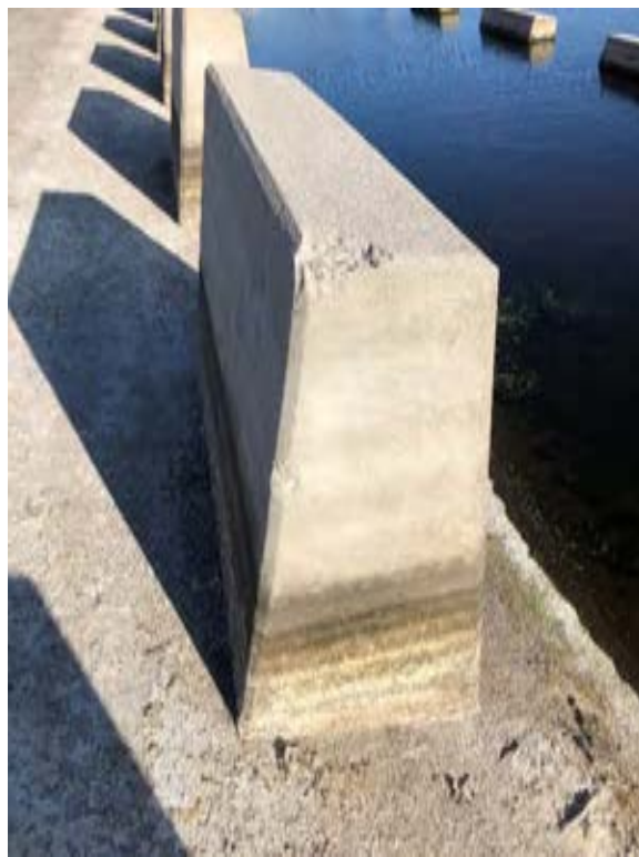
Photo 7 Superficial damage to baffle likely due to shooting
