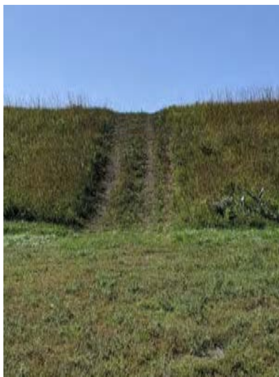
Photo 34 Vehicle tracks and rutting on downstream face of embankment
