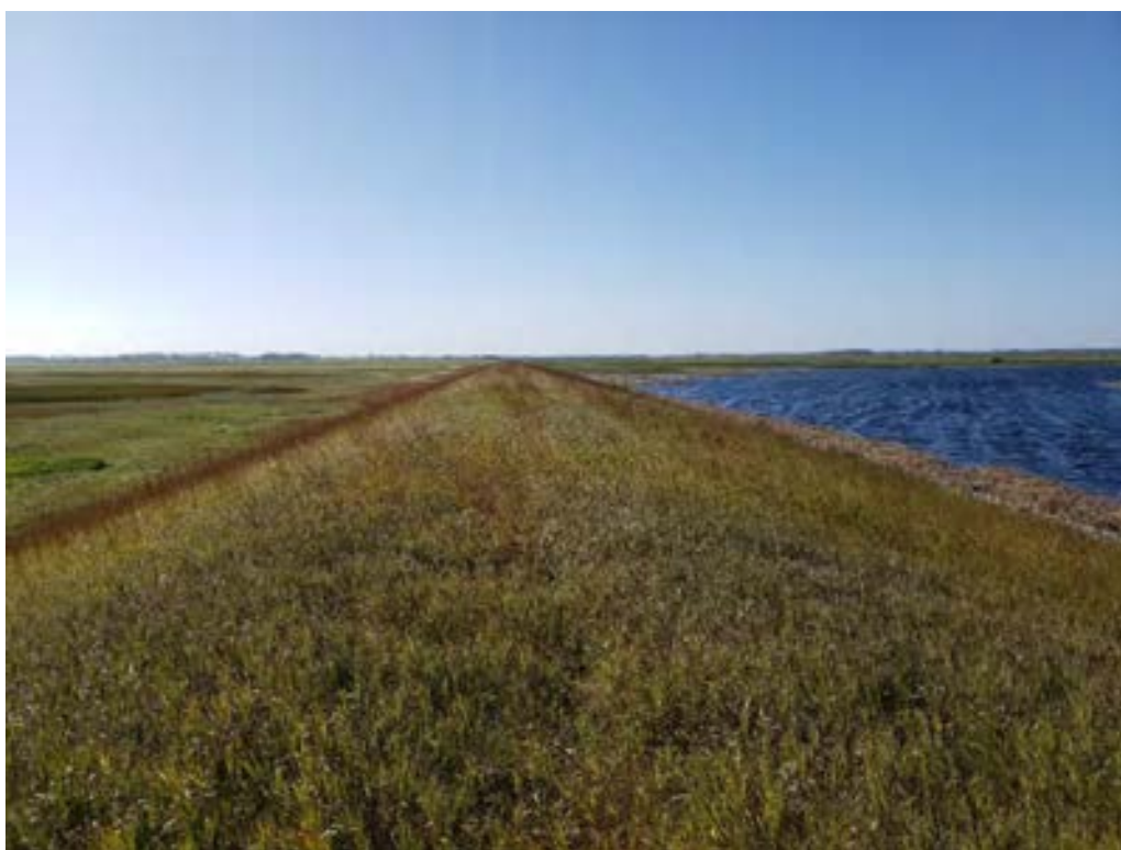
Photo 28 Crest of North/South right embankment
