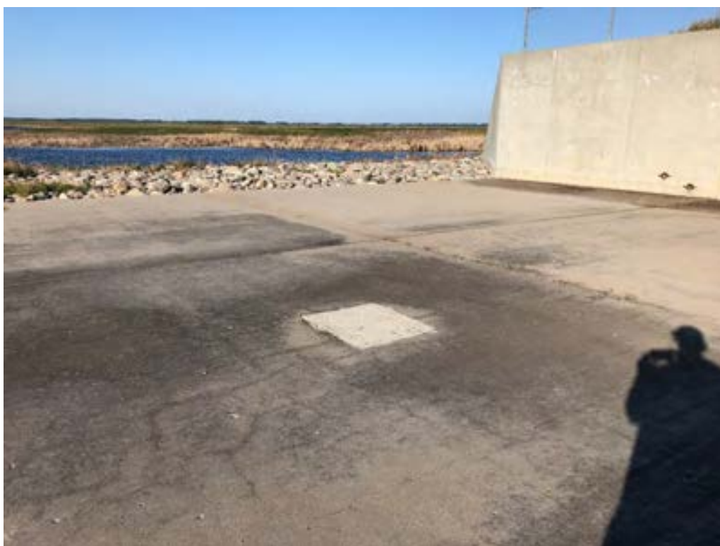
Photo 4 Concrete patch in floor of AS approach; patch is hollow and not adhered to surrounding concrete
