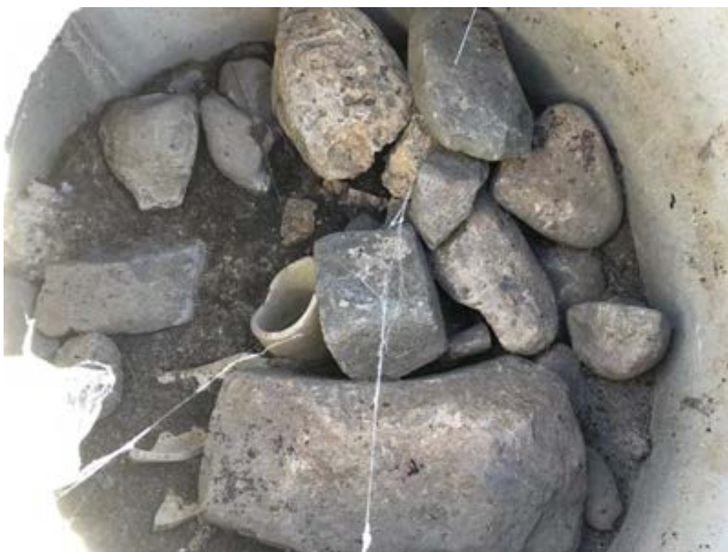
Photo 14 Drain cleanout broken due to vandalism by dropping rocks into manhole
