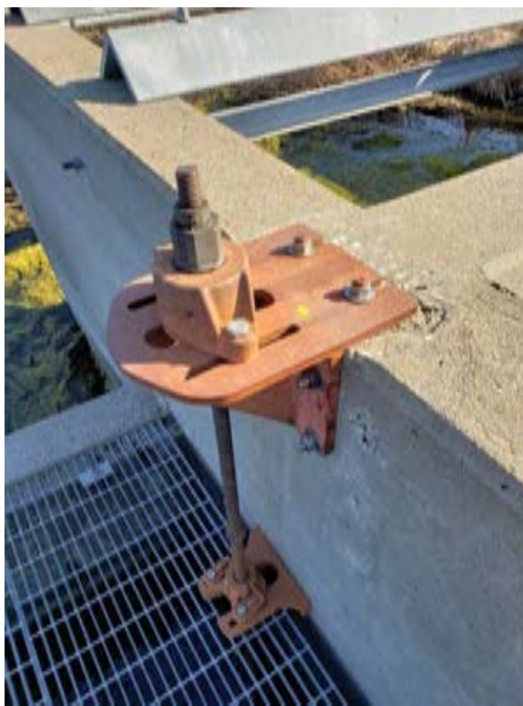
Photo 22 Low level drawdown gate operation mechanism; wheel is stored offsite
