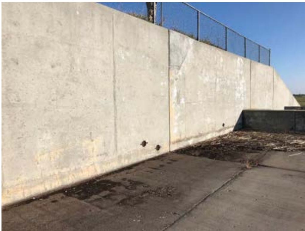
Photo 3 Left, upstream wall of auxiliary spillway; concrete patch located at Joint 5 of wall
