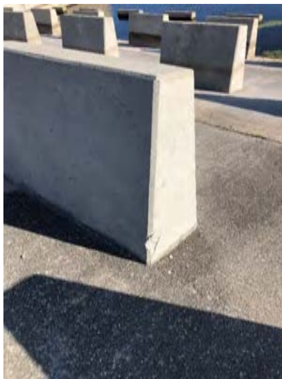
Photo 8 Superficial damage to baffle likely due to shooting
