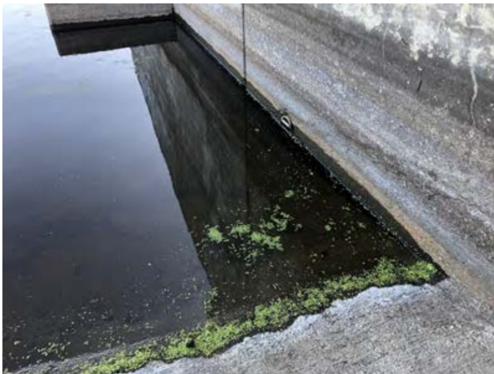
Photo 17 Lower auxiliary spillway foundation drains submerged due to improper drainage of stilling basin
