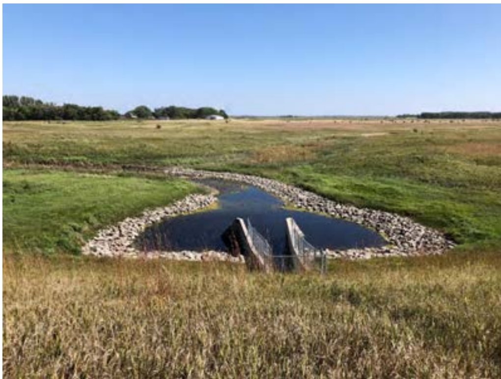
Photo 23 Plunge pool at the PS outlet; proper drainage is impeded by sediment and vegetative growth
