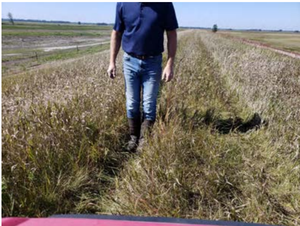
Photo 35 Vehicle rut on crest of dam
