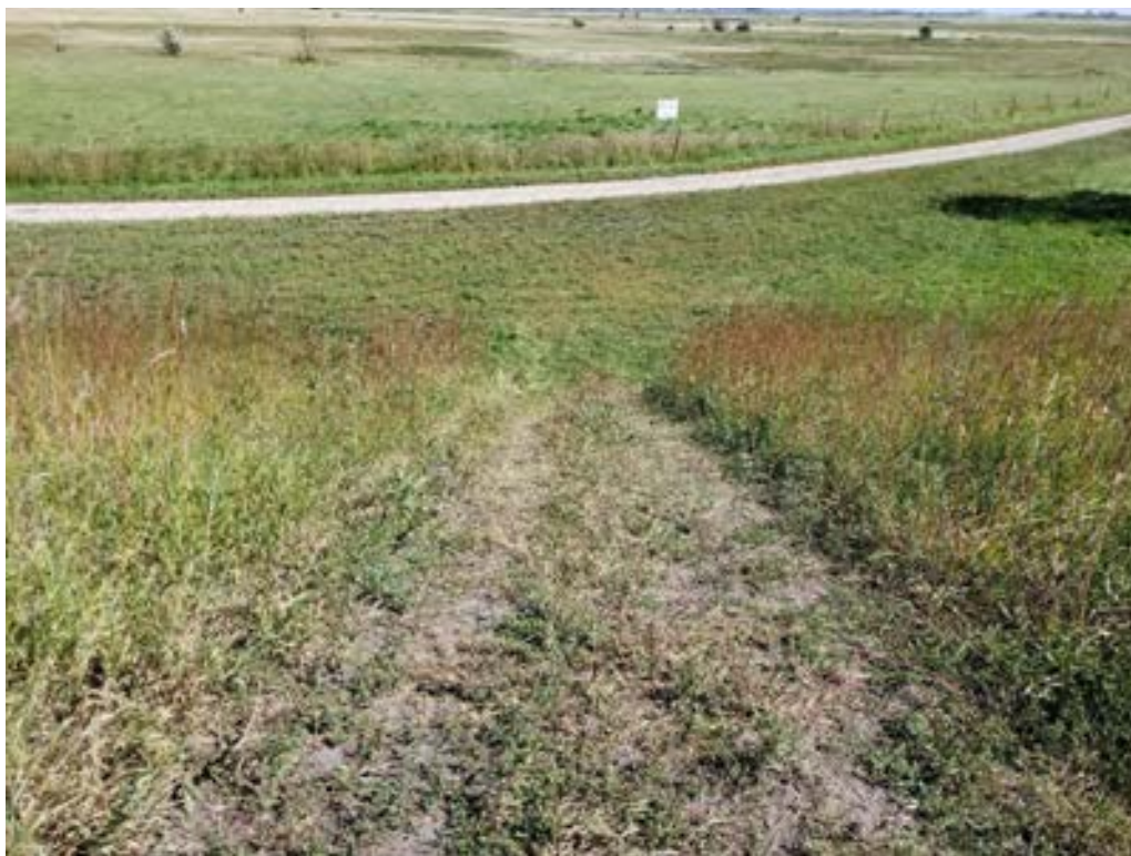
Photo 31 Worn vehicle tracks on downstream face of embankment
