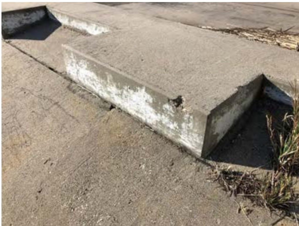
Photo 9 Damaged edge of auxiliary spillway crest weir
