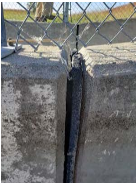
Photo 25 Joint separation of PS outlet wall; waterstops appear to be intact
