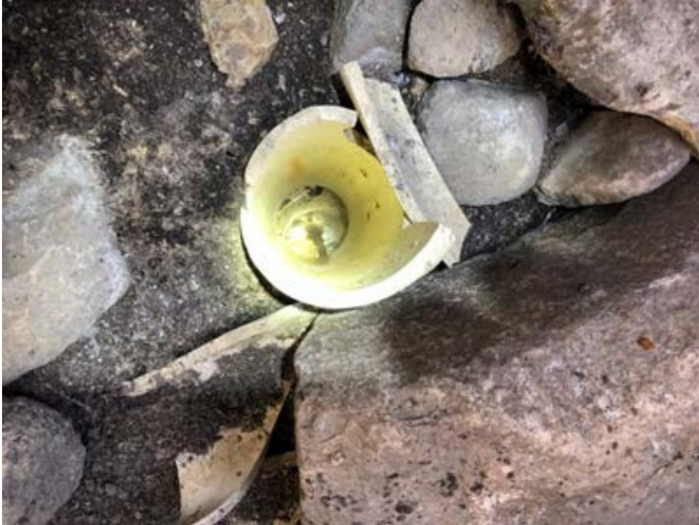
Photo 15 Broken drain cleanout dislodged from foundation drain pipe
