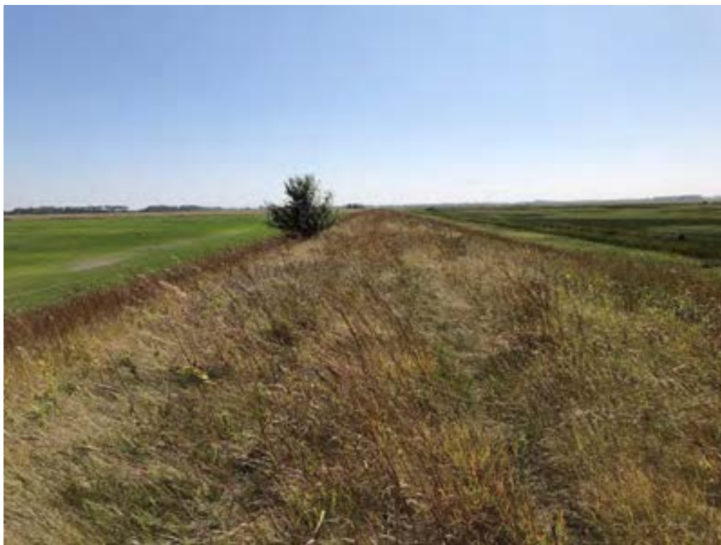
Photo 29 Crest of North/South right embankment
