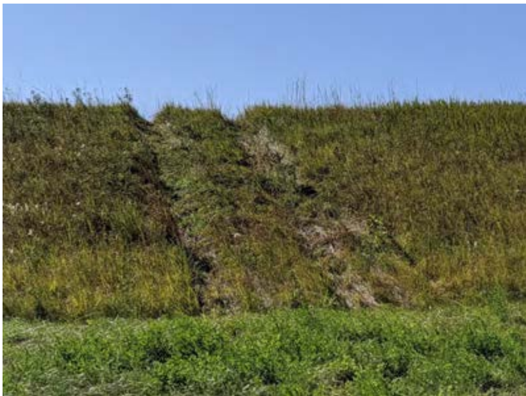
Photo 33 Vehicle tracks and rutting on downstream face of embankment
