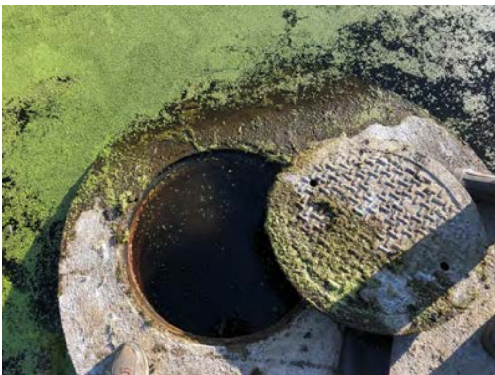
Photo 12 Drain access manhole submerged in stilling basin of auxiliary spillway
