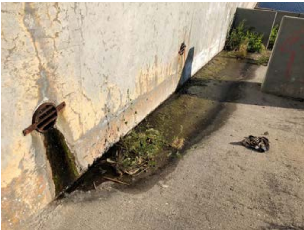
Photo 16 Auxiliary spillway foundation drains functioning; heavy vegetative growth
