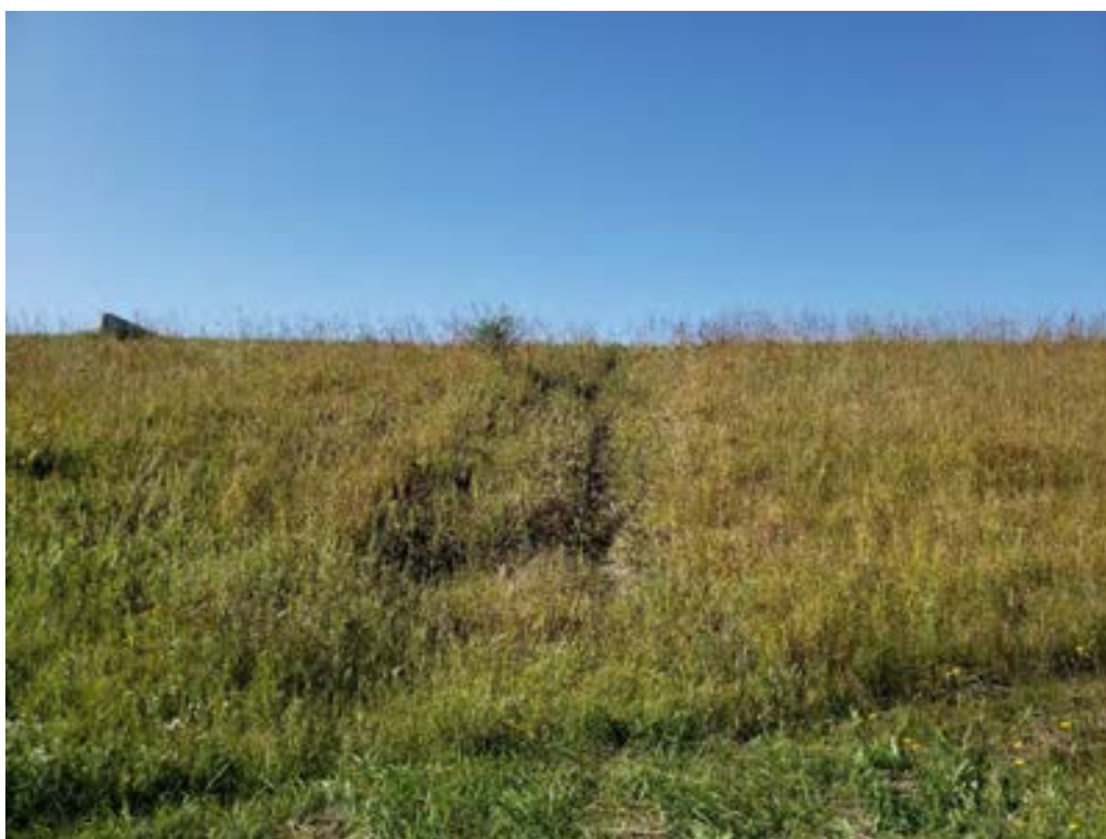
Photo 30 Erosion on downstream face of embankment near left wall of auxiliary spillway
