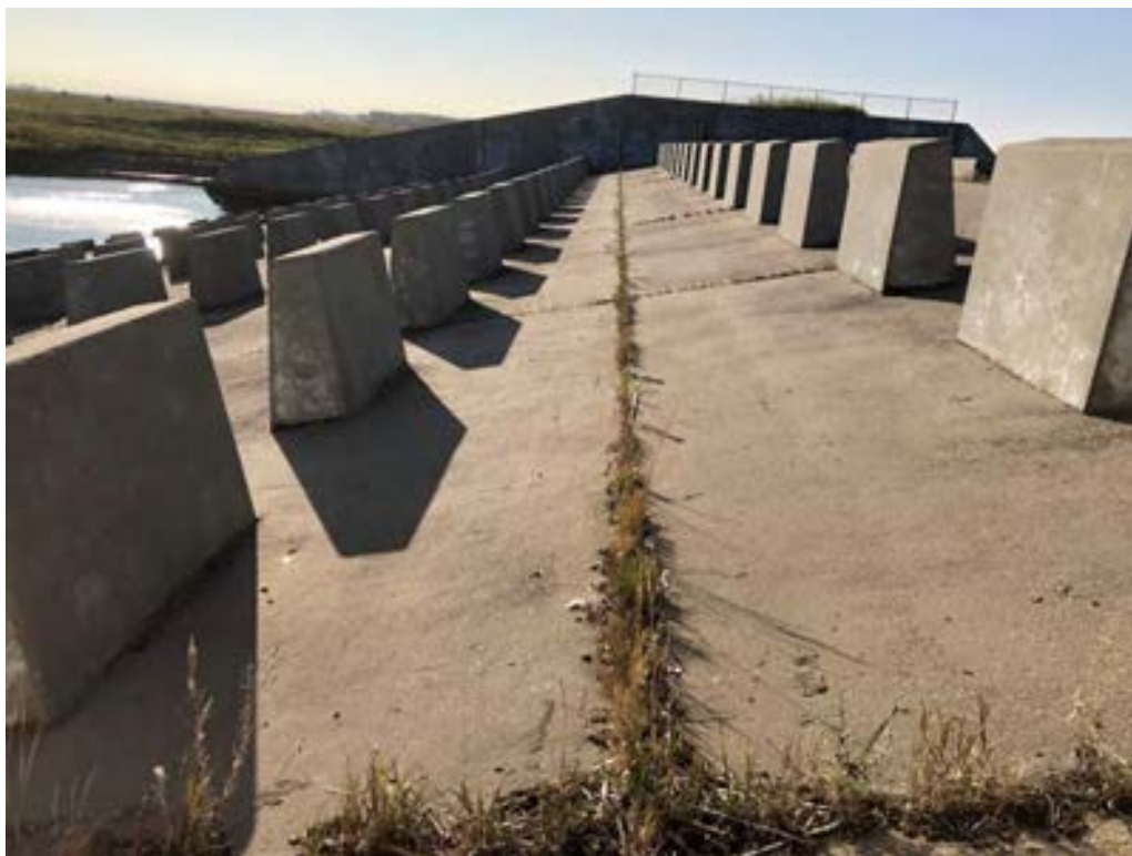
Photo 5 Heavy vegetation in floor joint of auxiliary spillway
