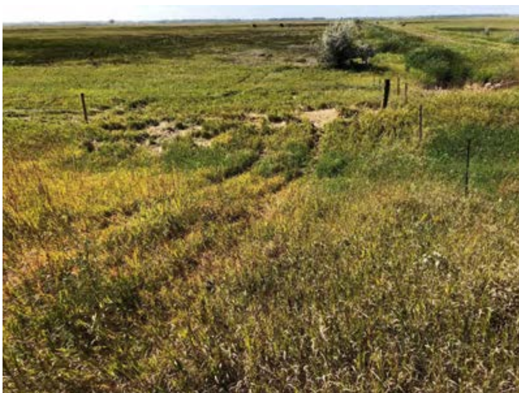
Photo 32 Vehicle tracks on upstream face of embankment
