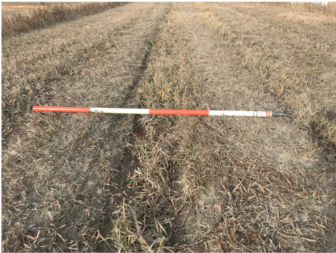
Photo #3 - View of Vehicle Rutting upon Dam Crest
