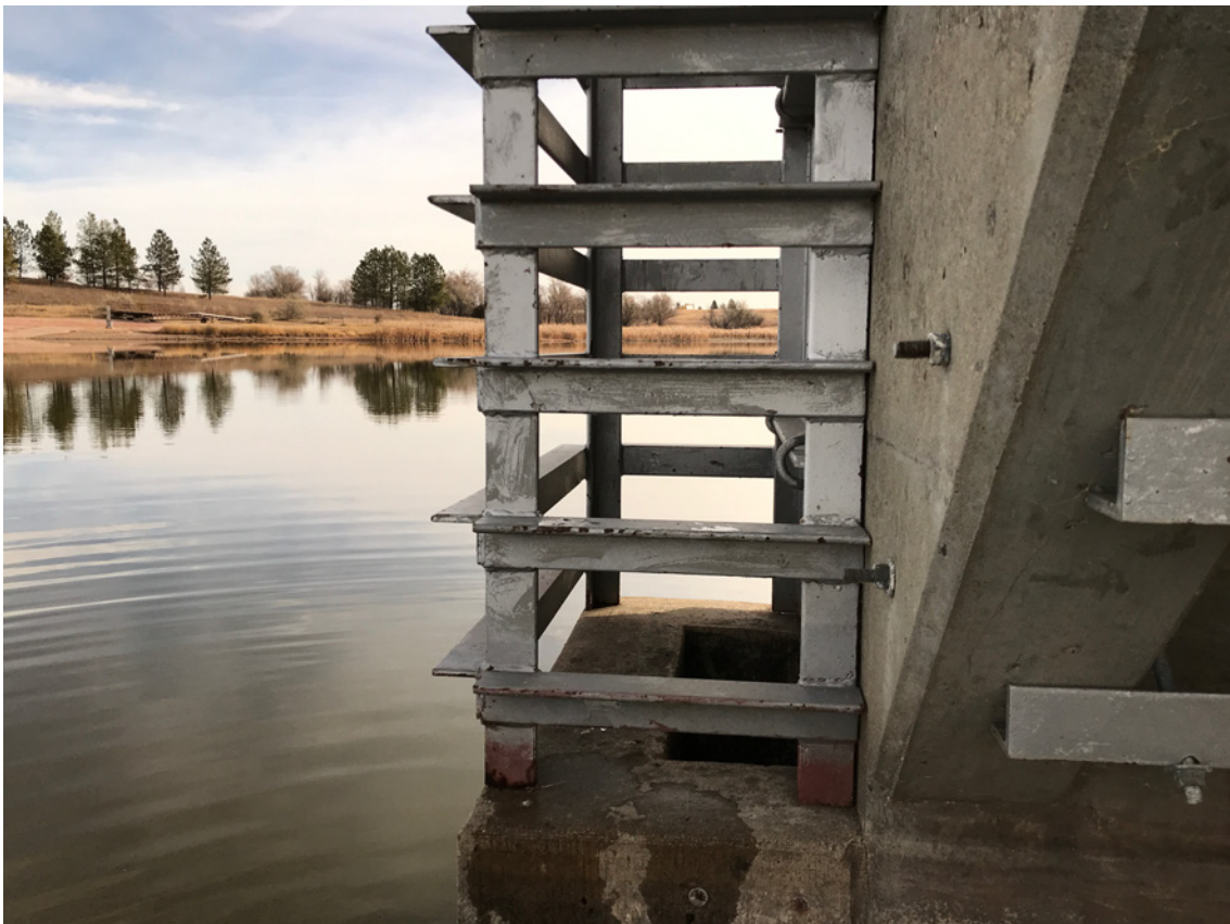
Photo #24 - View of Stage-1 Inlet Trash Rack
