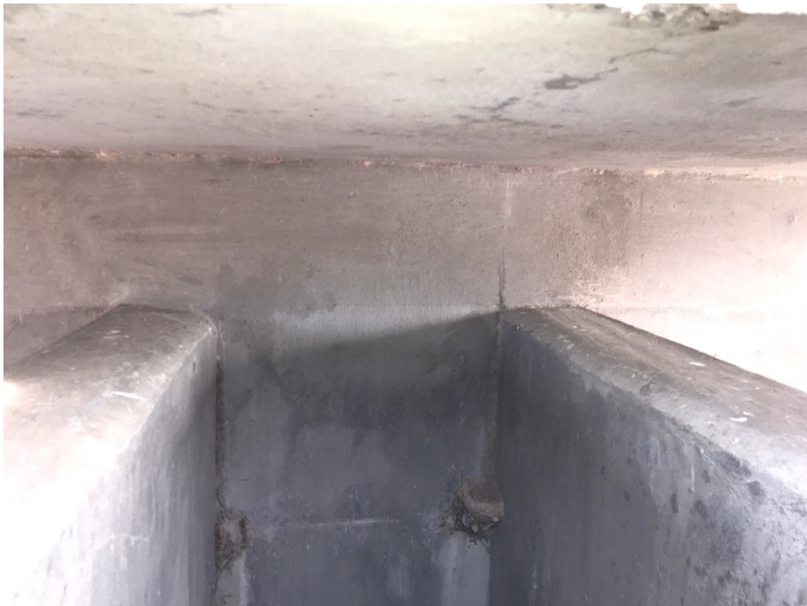
Photo #18- View from Stage-2 Inlet Orifice from within Riser Tower Structure
