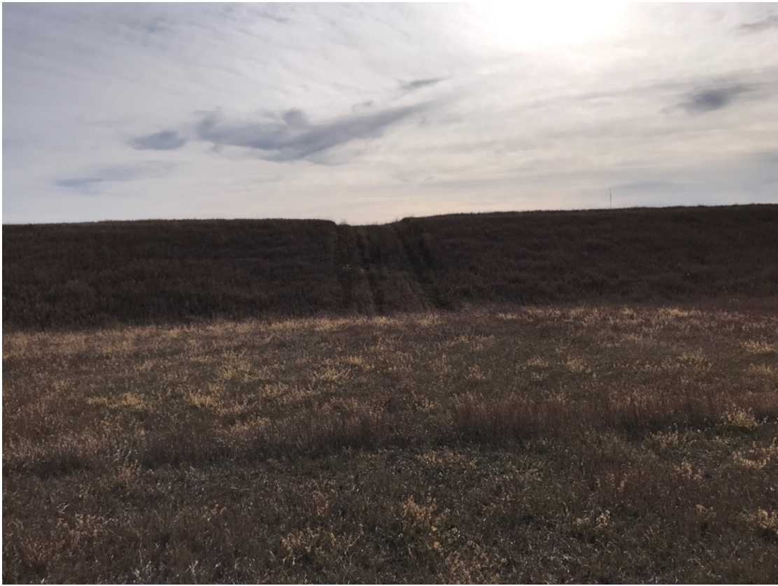
Photo #49 - View of Sod Chute on Auxiliary Spillway with Apparent Vehicle Tracks
